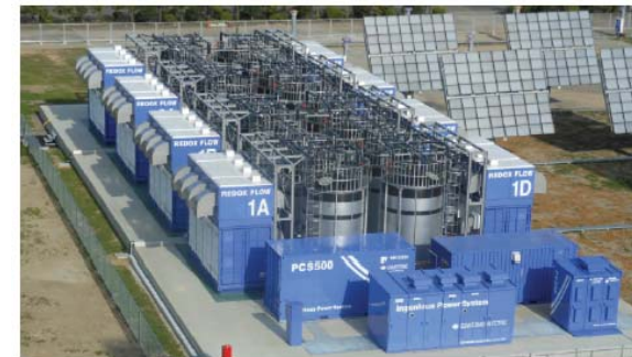
Aerial view of the 5-MWh RFB and 100-kW PV.
