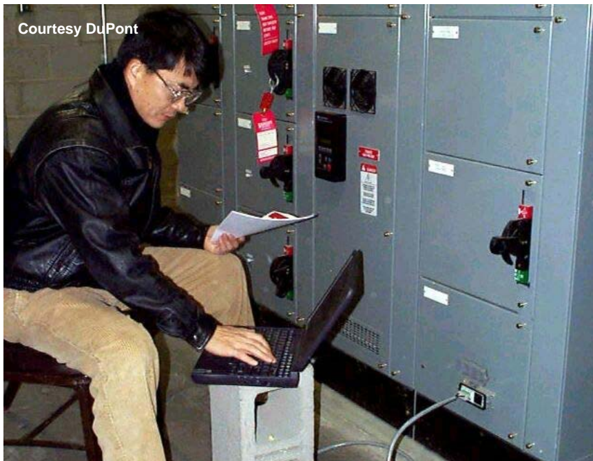
Smart MCC troubleshooting
