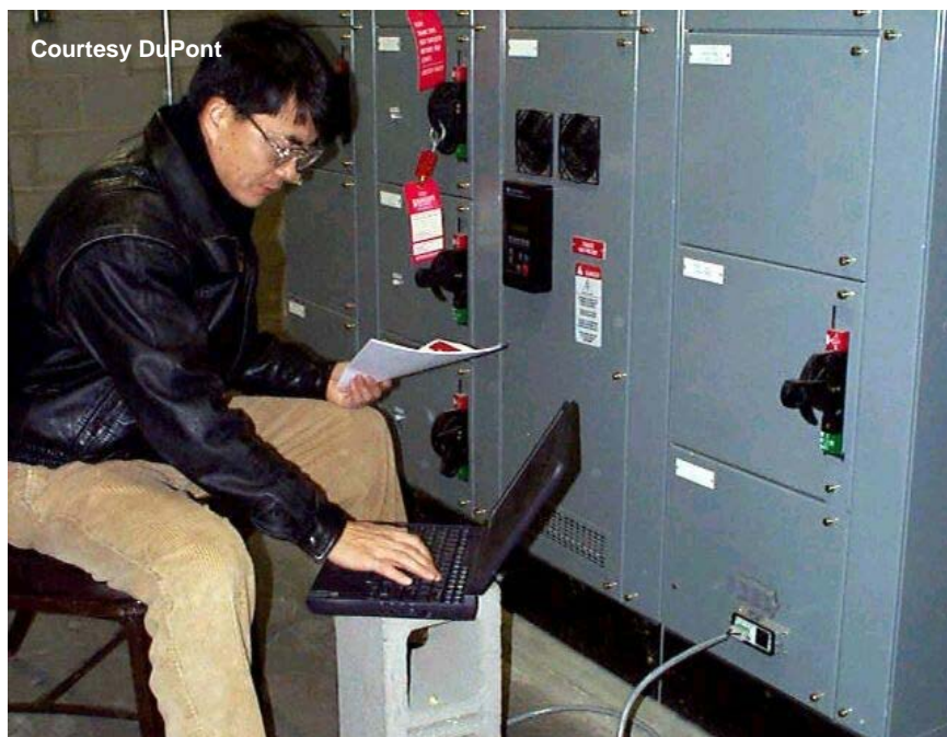
Smart MCC troubleshooting
