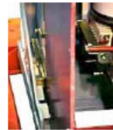
3. Circuit Breaker & Tray Latched in Place
