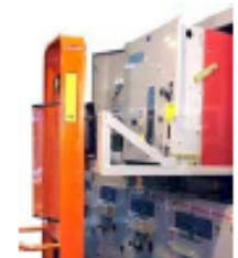
6. Roll Circuit Breaker in Cell
