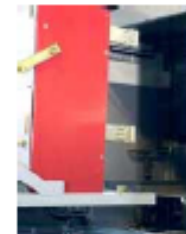
5. Circuit Breaker Approaching Hook
