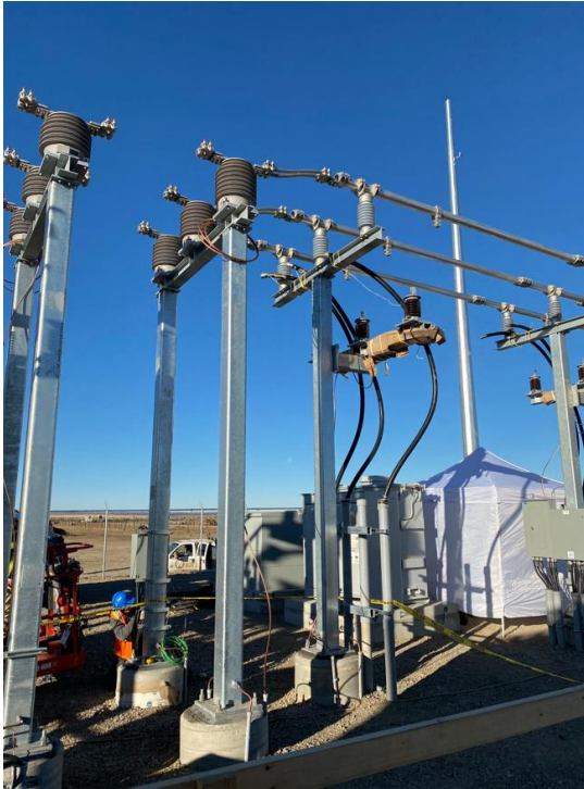
Overhead connection to metalclad breaker
