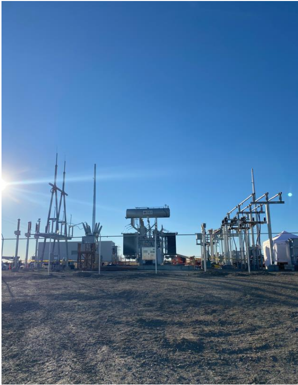
Substation is currently on operaticon since January 2021
