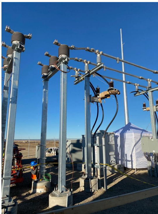
Overhead connection to metalclad switch
